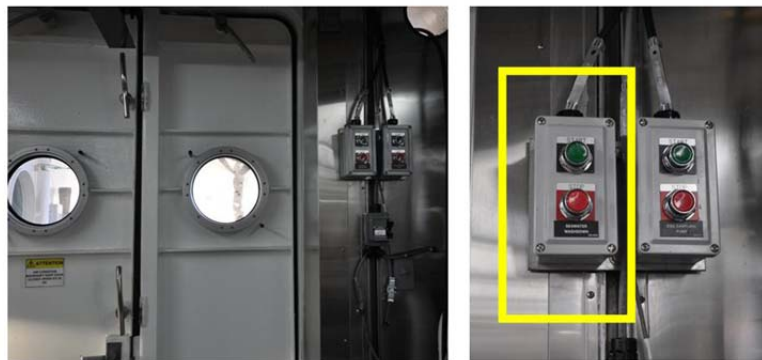
Figure 2. On/off for HPU seawater washdown is located in the wet lab near the doors to the side-sampling station.
