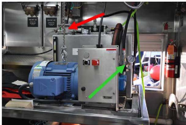
Figure 1b. Photo of HPU (with roll-up door behind it). The black button is the START, the red button is the STOP. The green arrow points to the pressure gauge. The red arrow points to the temperature gauge for the hydraulic fluid.
