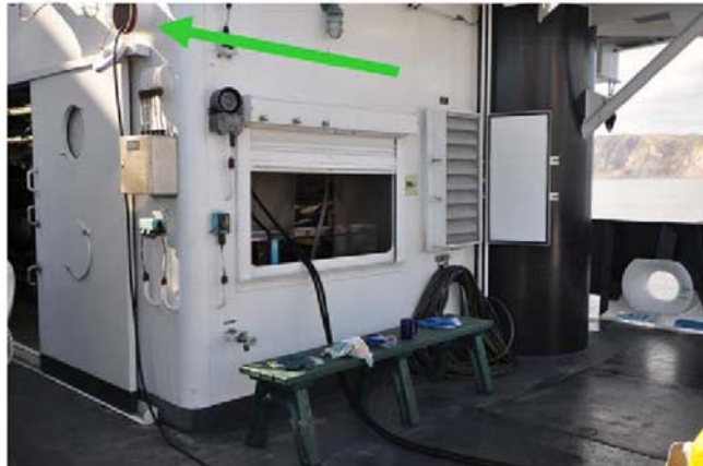
Figure 1a. Photo from fantail of aft entrances to wet lab. The HPU hoses are currently run out of the roll-up door. The green arrow points to the bulkhead opening which would be the preferred route for the HPU hoses.
