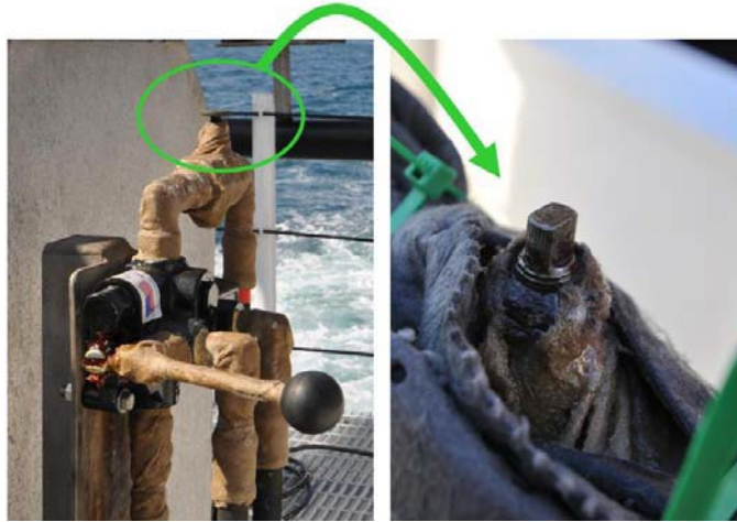
Figure 3. Photo of Winch Speed Adjuster (prior to failure) and close up of poor screw condition and leak.
